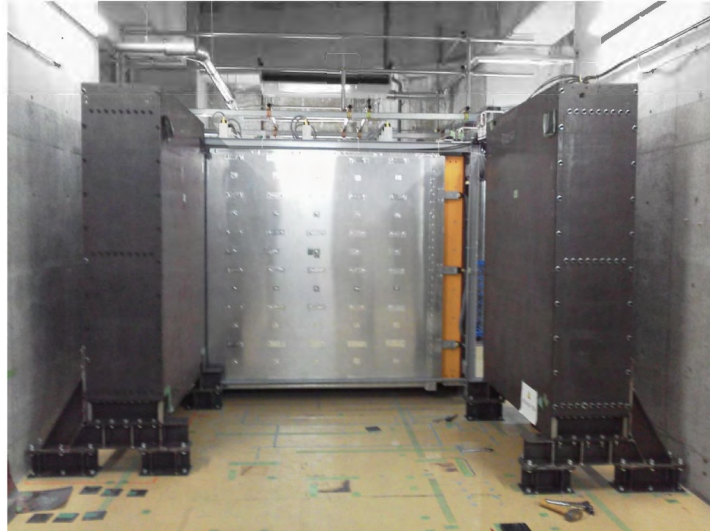
(b) Wall-MRDs installed in B2 floor.
