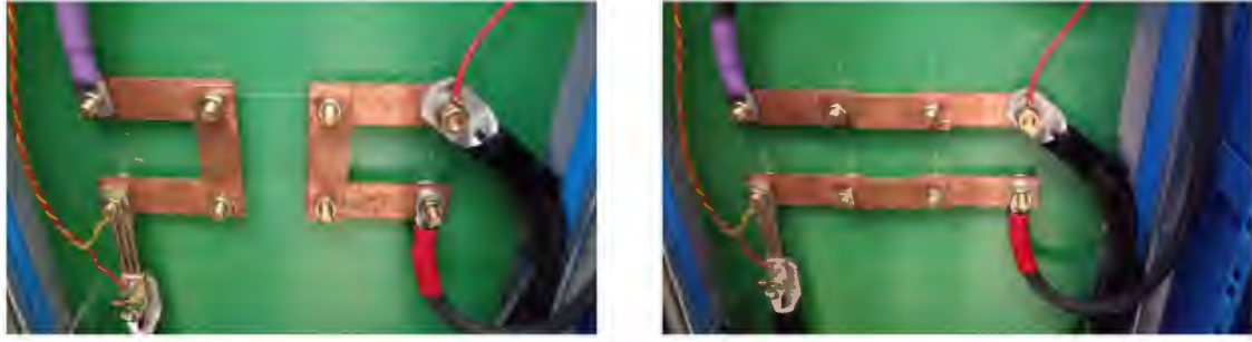
Figure 4-14: Panel for switching magnet current in forward (left) and reversed (right) mode.
