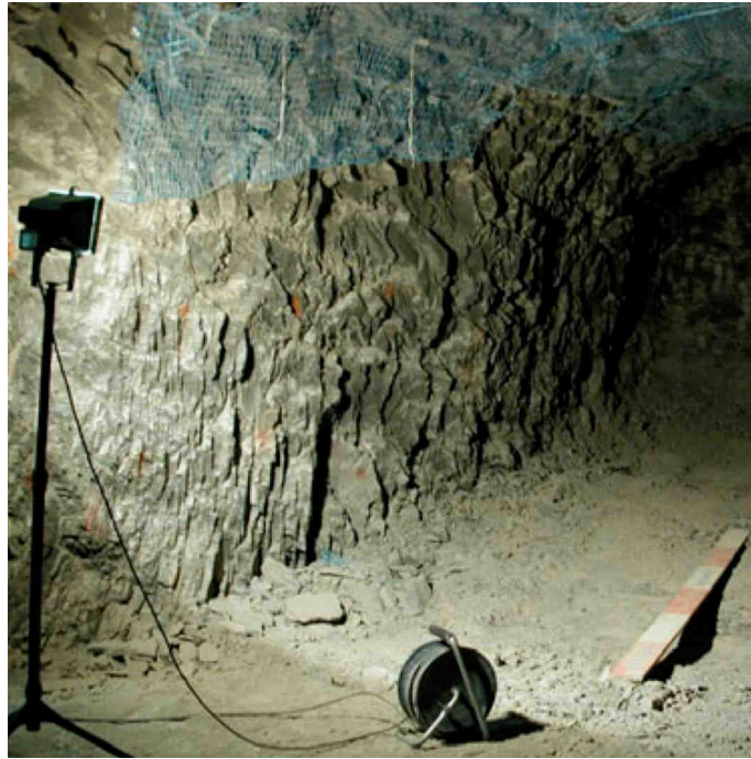
Figure A.4-19. Intense extensional EDZ fracturing in the sidewall of the Mont Terri URL Photo: B. Niederberger
