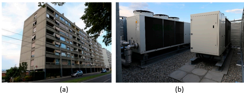
Figure 2. Monovalent ASHP system. (a) non-retrofitted MFB and (b) industrial ASHP on the roof with sound-proofing wall panels.
