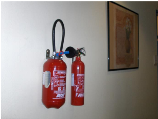
Fig.6: “Conversation between two fire extinguishers” (D2) SINGLE-COLUMN FITTING IMAGE
